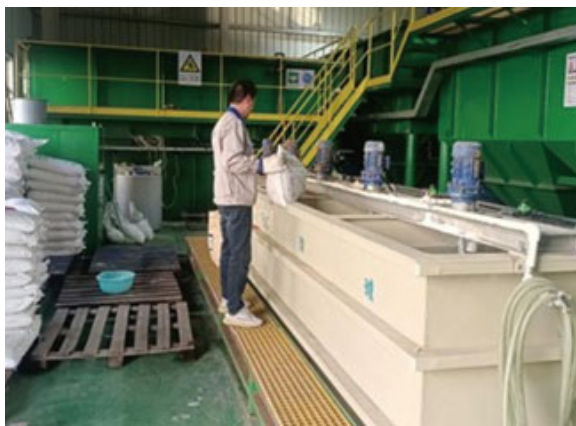
Waste Water Treatment in Action
