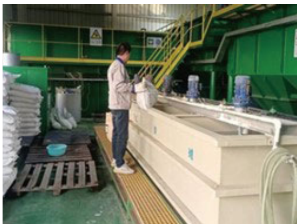
Waste Water Treatment in Action
