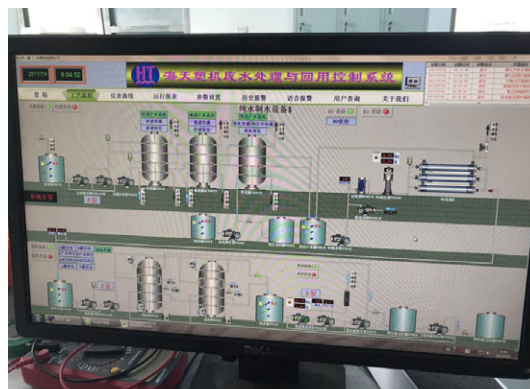
Waste Water Treatment and Reuse Control System
