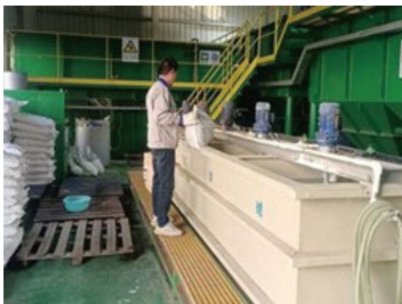
Waste Water Treatment in Action
