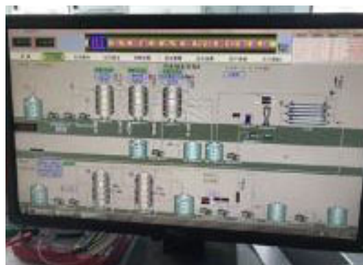
Waste Water Treatment and Reuse Control System
